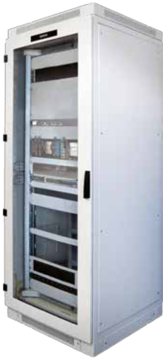
■ Telecommunication engineering cabinet at a 110kV station
