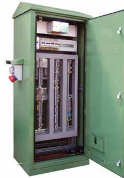
■ 110kV bay cable cabinet with a measuring system
