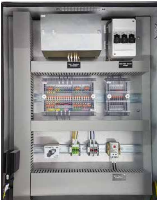
→ Equipment of the measuring circuits cabinet
