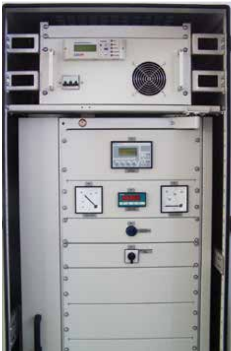
→ Inverter / PSU mounting and custom height swing frame
