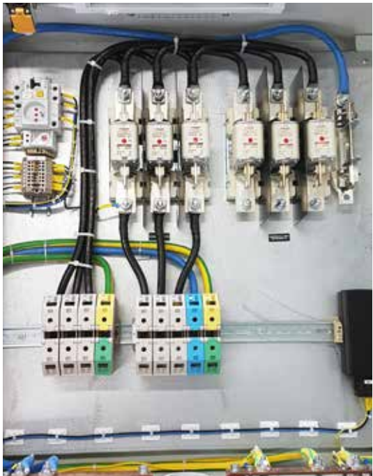
→ Equipment of an intermediary cabinet
