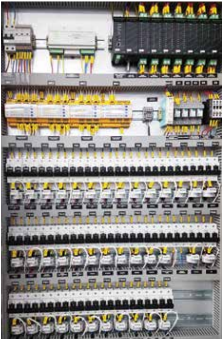
→ The controller and the earth fault control system for the PW 220V DC cabinet
