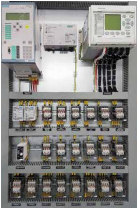
→ Digital protection equipment mounted on a switchgear mounting plate
