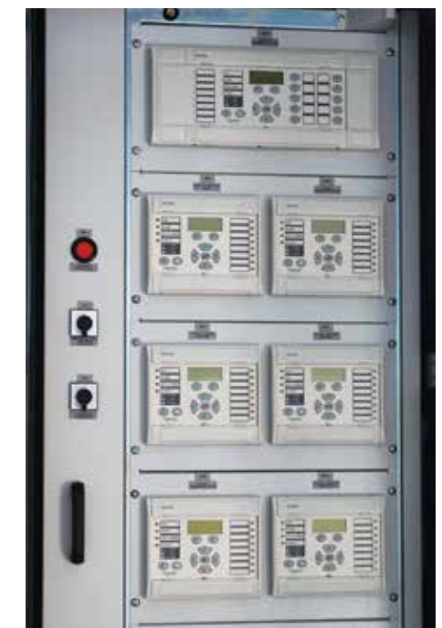
→ 110kV bay protection mounted on a swing frame
