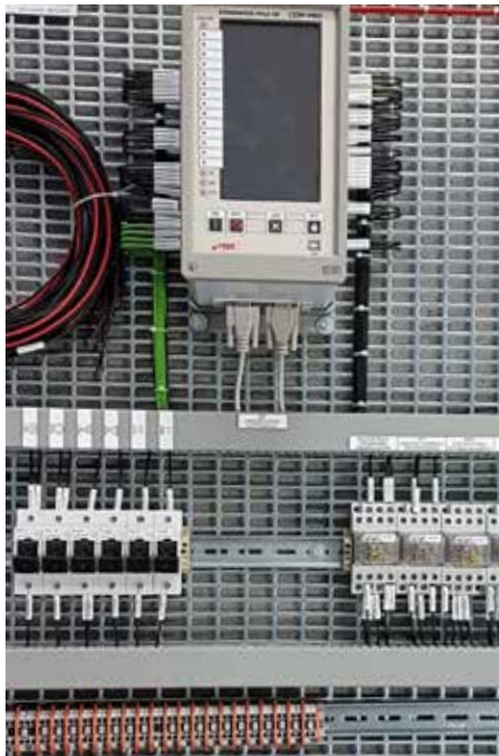
→ 15kV switchgear cell plate
