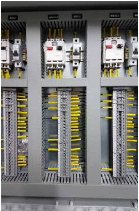
→ Equipment for the facilities switching station
