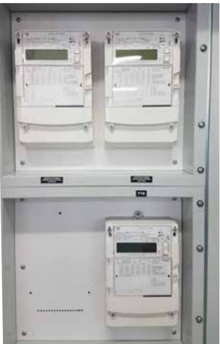
→ Metering devices fitted into the meter box
