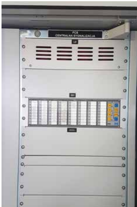
→ Signalling system with an acoustic circuit fitted inside the cabinet
