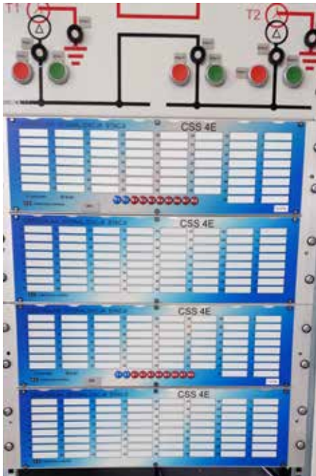
→ Station's central signalling system mounted within the local control cabinet
