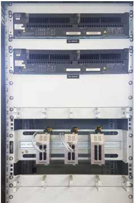
→ Active elements of the SUT cabinet equipment
