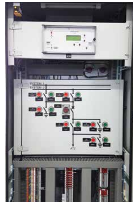
→ Tilt-plates for the control system and the circuit breaker controller, mounted in the FS-1 cabinet
